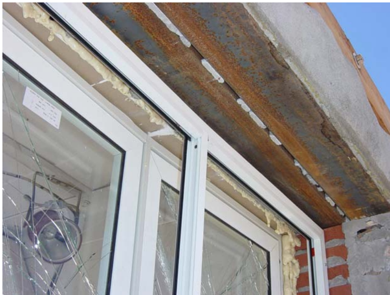
Figure 9. Post-Test Photo of Frame Deformation.
