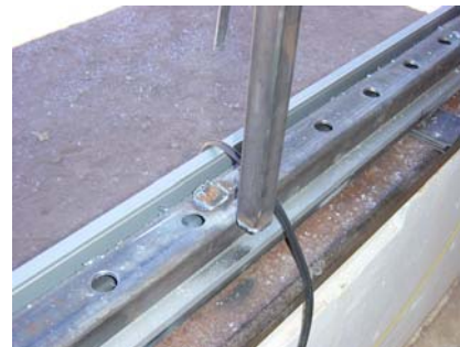
Figure 6. Failure of Standard Muntin End Connection.
